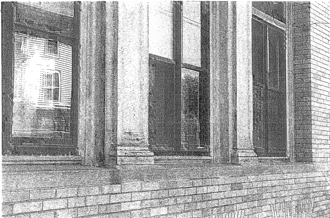
TYPICAL PALLADIAN WINDOW METAL TRIM NOTE RUSTING
