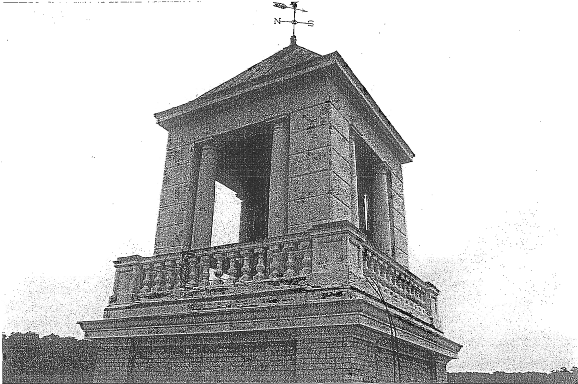
OPEN BELL LEVEL FROM ROOF OF BUILDING NOTE DETERIORATING PAINT CONDITION
