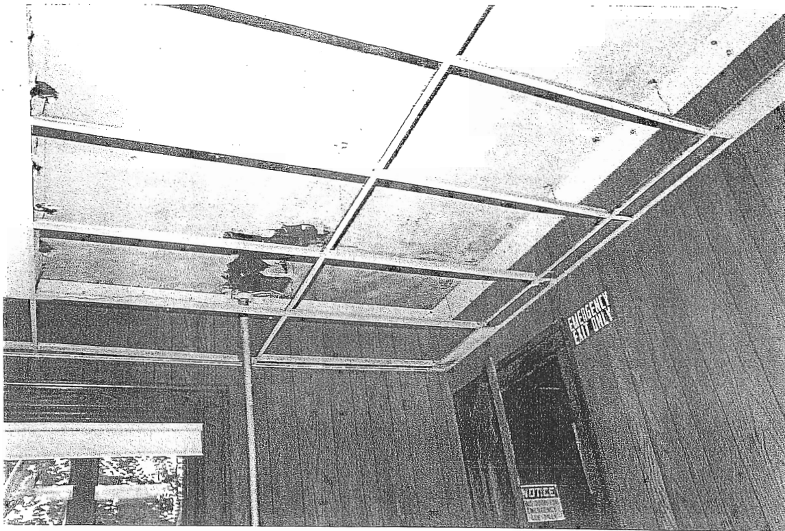
MEMORIAL HALL - PARTLY DISMANTLED ACOUSTIC CEILING EXISTING - DAMAGED PLASTER CEILING ABOVE
